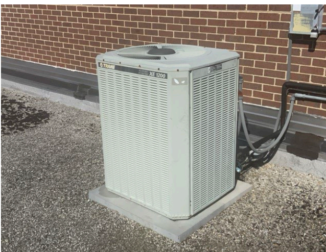
17 - SPLIT SYSTEM CONDENSER
