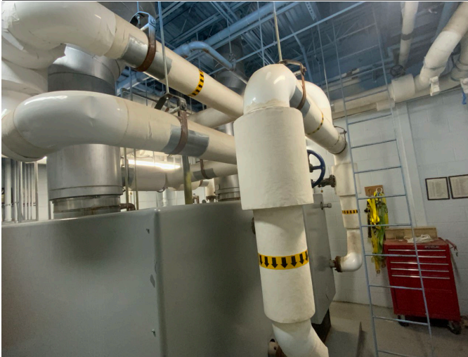
19 - HVAC PIPING SYSTEM
