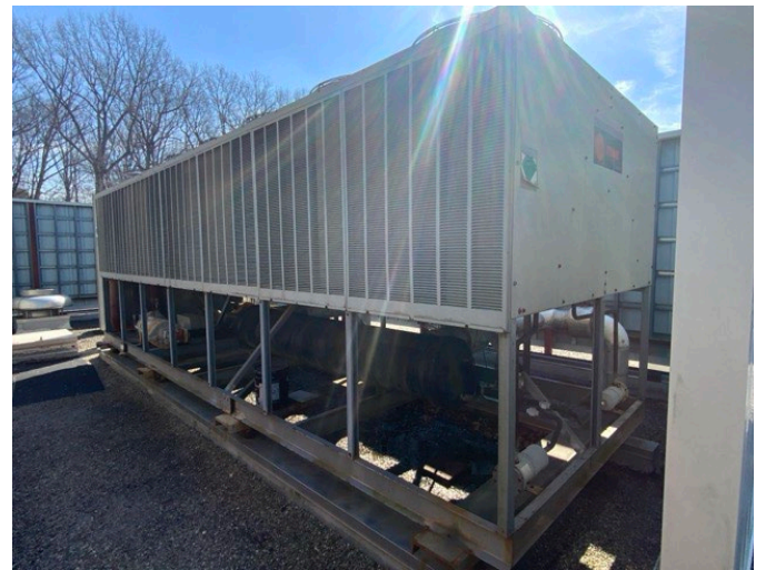
16 - AIR COOLED CHILLER
