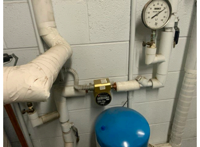
14 - PLUMBING SYSTEM PIPING
