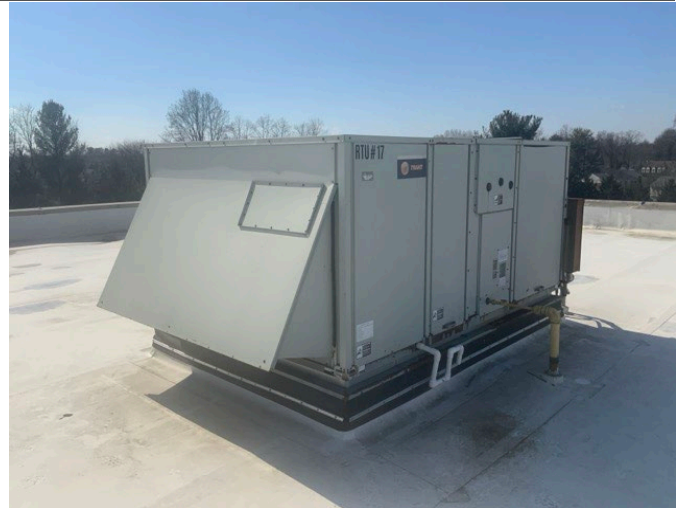
20 - ROOFTOP PACKAGED UNIT
